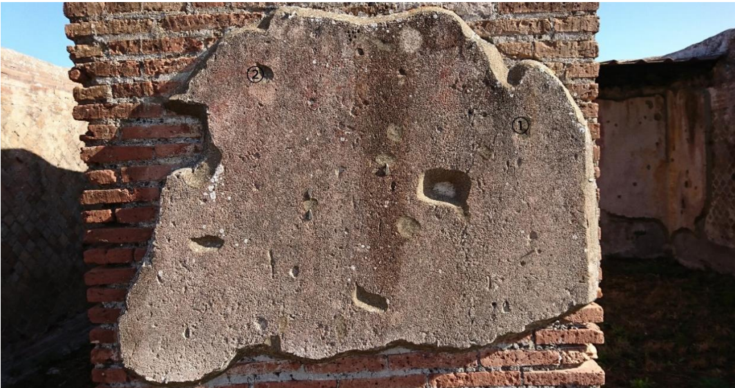
Fig.15 North wall of 15-9 (Entrance of 7)
